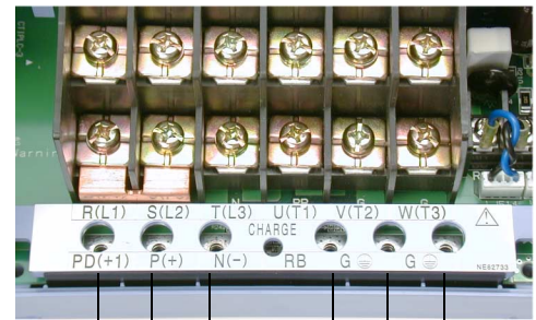
Retention screws locations for capacitor bank
